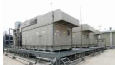
Aeon's private power generators
