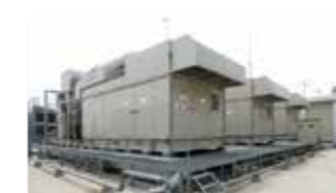
Aeon's private power generators
